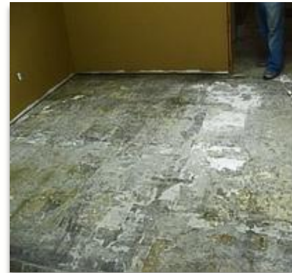
Slab with asbestos adhesive
